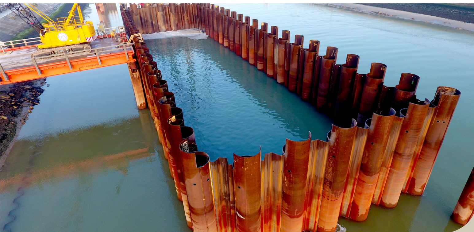
Installed tubular combined wall from the water, Nieuwpoort — Belgium © Werf Stormvloedkering Nieuwpoort — THV Herbosch-Kiere — Jan De Nul
